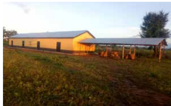
Construction of three classroom block and an office at Koshim community in the Northern Region
