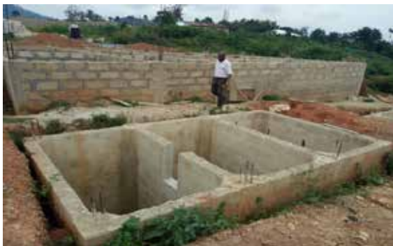
The 10-Unit toilet facility for Anpampatia, Atiwa West District, passes footing level
