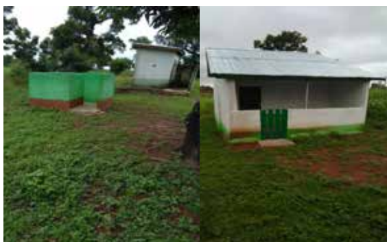
Construction of Maternity Block with washroom at Gupanarigu Community in the Northern Region
